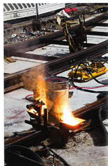
FIGURE 2.6.1b: The thermit reaction is useful in repairing or joining together railway tracks. The extreme heat melts the iron, which then runs into any cracks and fills them.
